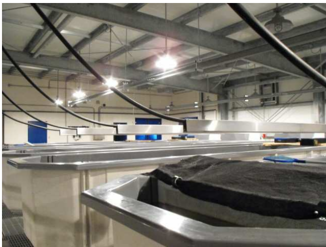
Food is blown to the fish down the black pipe and then directed across the whole tank by the aluminum trough.
