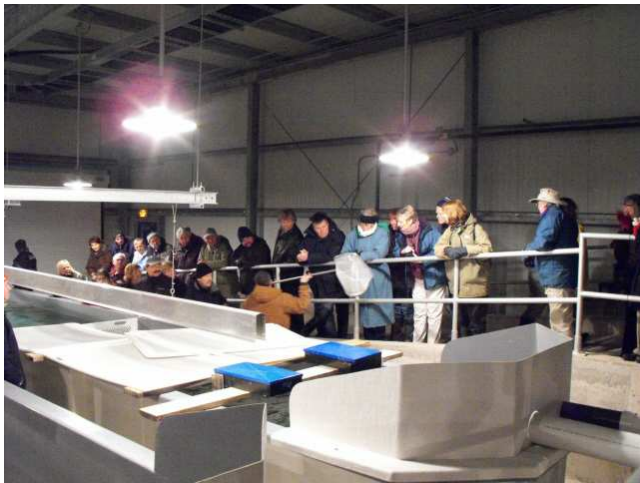
Inside the new substation on the Front Rd
